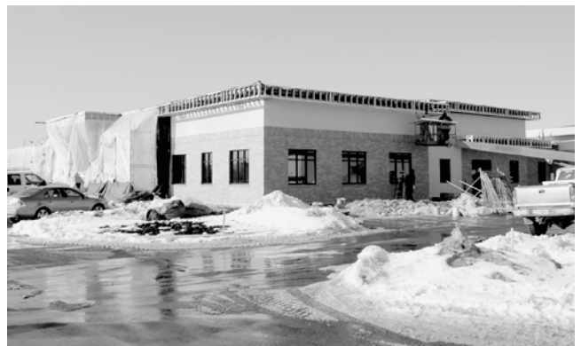
Data Dimensions' new state-of-the-art Tier 3 data center was designed and structurally enhanced to be capable of withstanding an F5 tornado.
