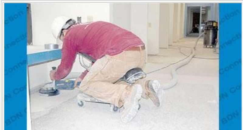
CCI worker Trent Austin polishes the floor at the former Beloit Library. The building renovations will be completed by July 2. Staff photo by Hillary Gavan
